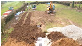
This page, clockwise from top: guests can enjoy a fresco dinner; the gold galleried hallway; the ostrich en suite bathroom; installing the new sanitation system
